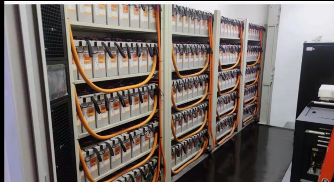
Uninterruptible Power Supply (UPS)
