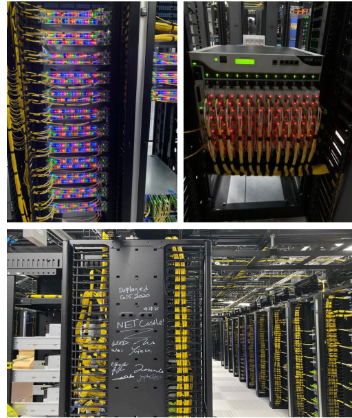
Figure 6: Netcastle Hardware Platform.
