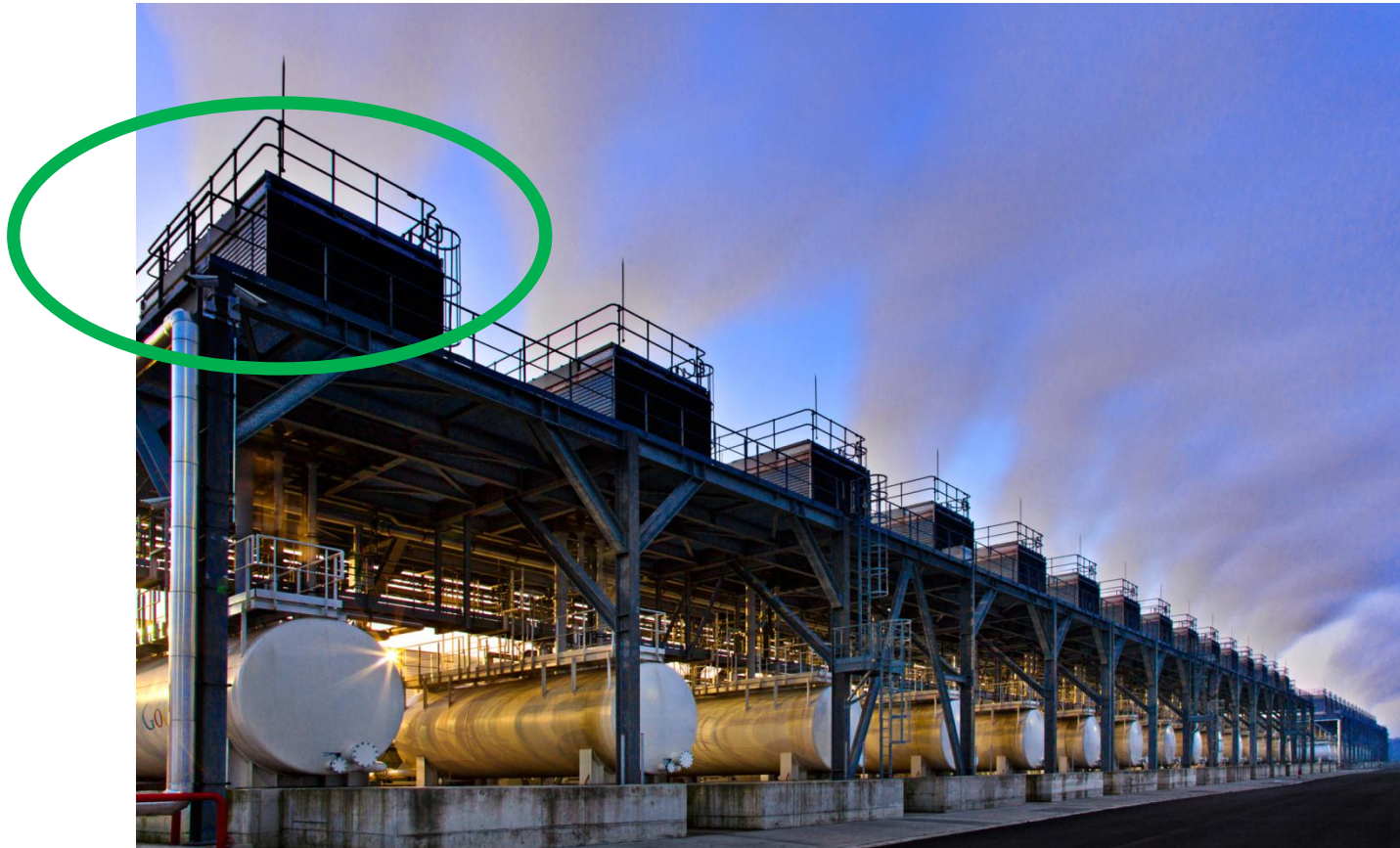
Cooling towers in Google's Belgium data center
