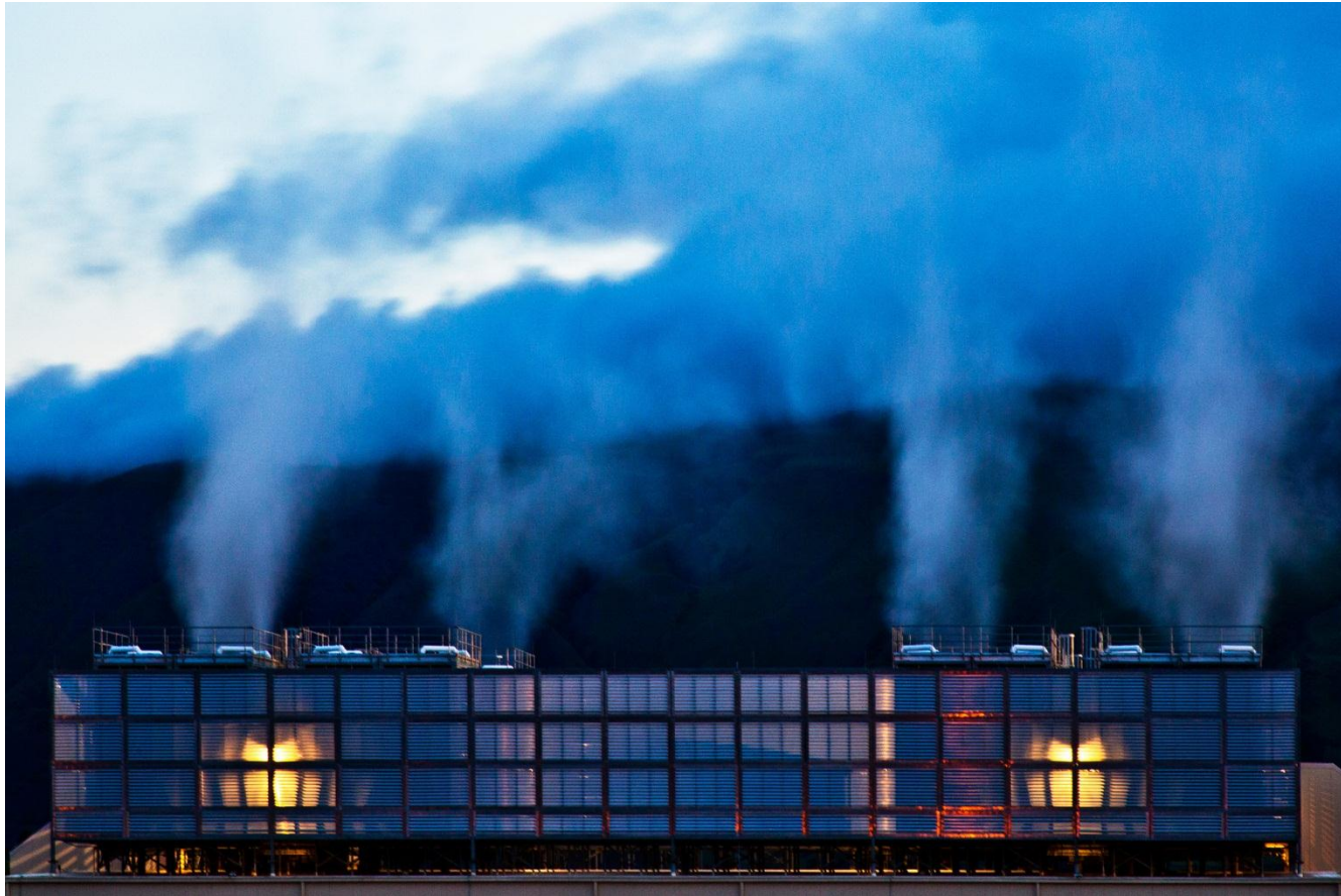
Water evaporation in Google’s Oregon data center
